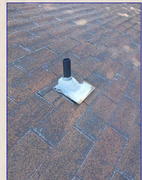
The Plumbing Vent(s)
