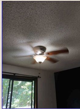
Ceiling fan operating
