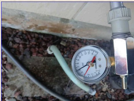
Hose bib operational.
