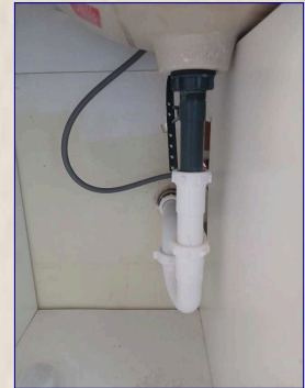
The bathroom plumbing view.
