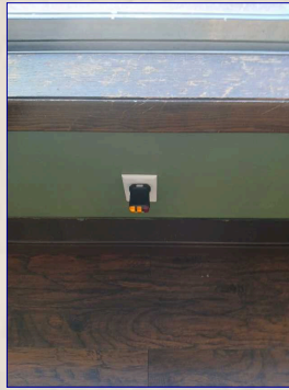
Electrical receptacle operating
