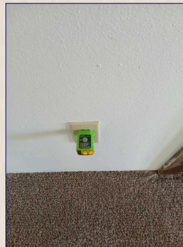
Electrical receptacle operating
