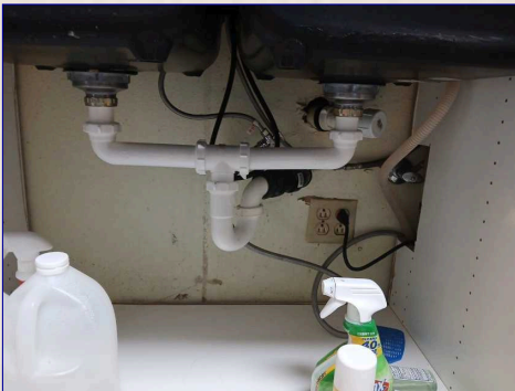
Kitchen plumbing view
