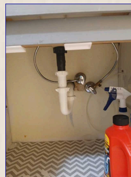
The bathroom plumbing view.
