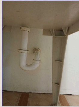
Laundry plumbing view.
