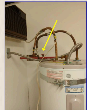
The Water Heater Water Shut Off Valve
